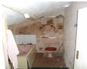
Poor living conditions found in some private housing
